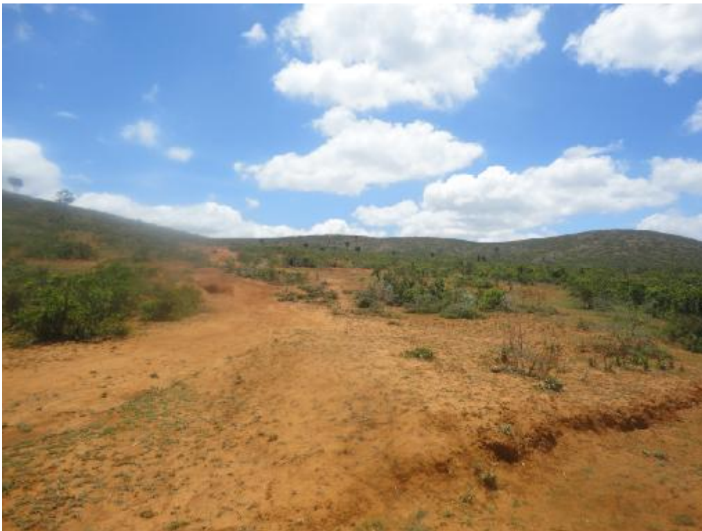
Damaged areas on Lusoi Hill – damages due to soil erosion
